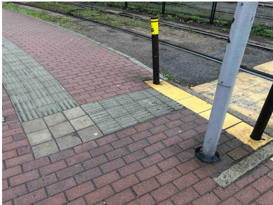
Picture 25. Textured surface and yellow markers for people with visual impairments. Photo: Jörgen Lundälv
